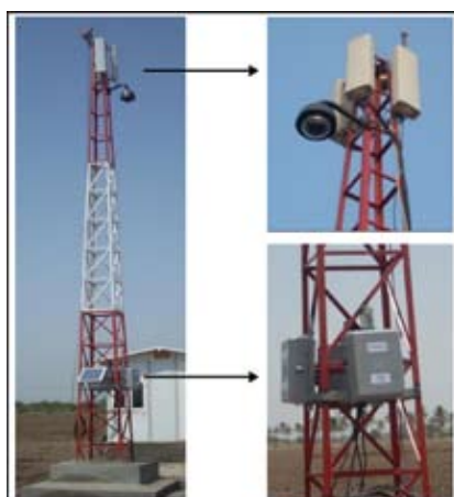
Fig 4: The receiver tower with PTZ camera and various monitoring units/devices
